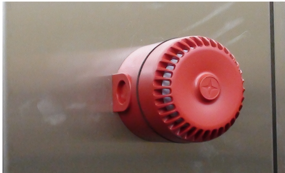
Figure 166: Signal horn on the valve manifold
