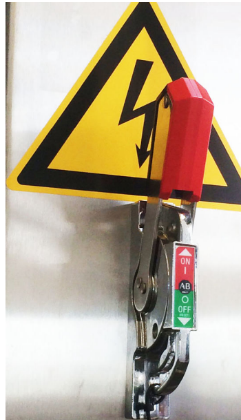
Figure 195: Main switch for the power supply on the switch cabinet
